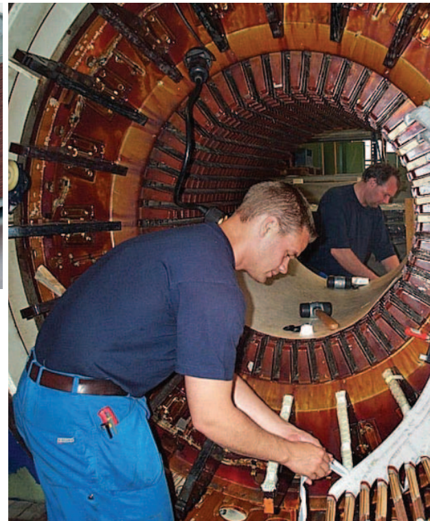
We take pride in being a complete supplier, irrespective of the complexity or size of the project.
